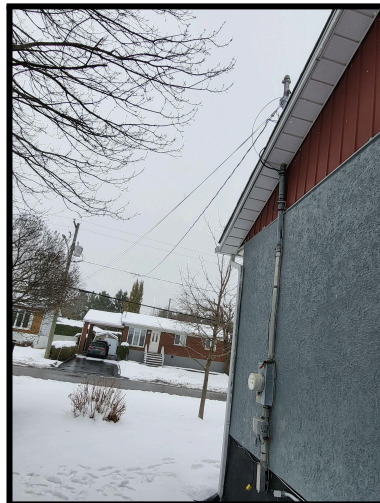
The Overhead Service
