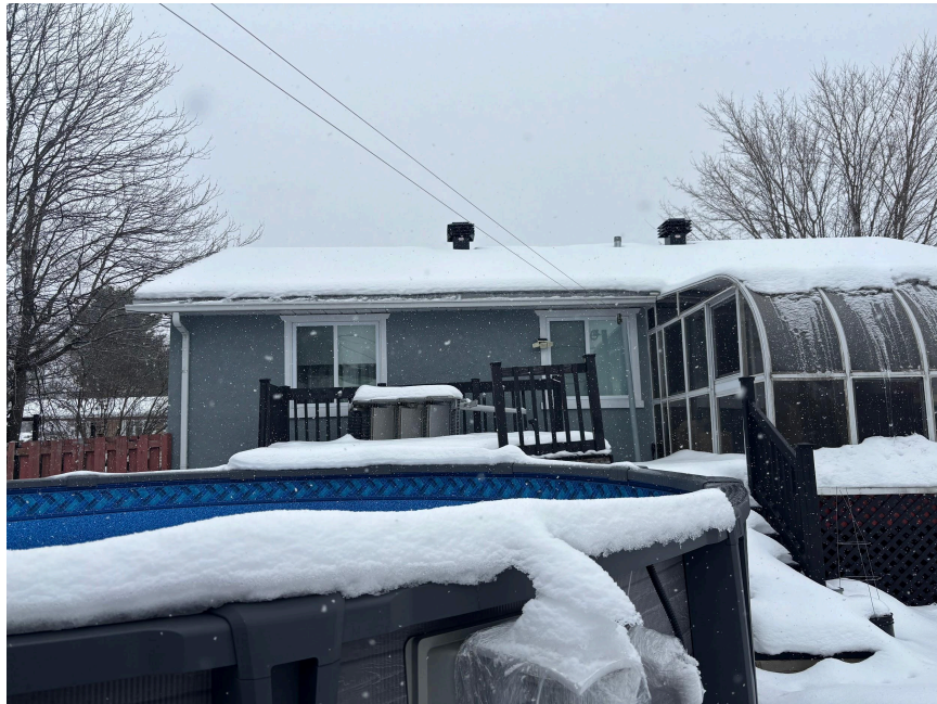
View of the roof at the south side of the house (backyard)
