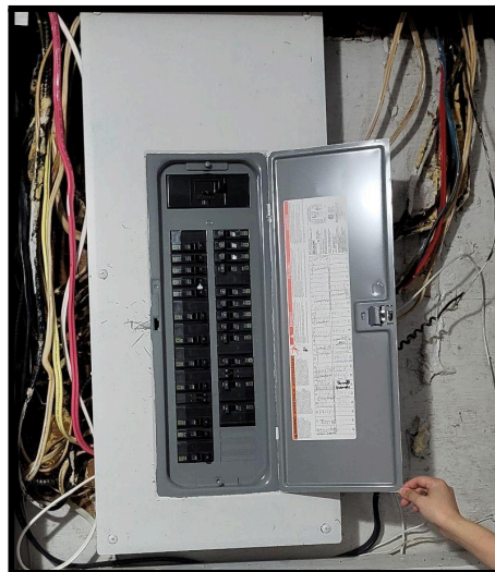
The Branch Wiring
