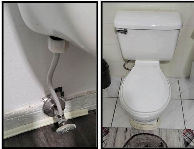
Toilet and the Shut Off Valve
