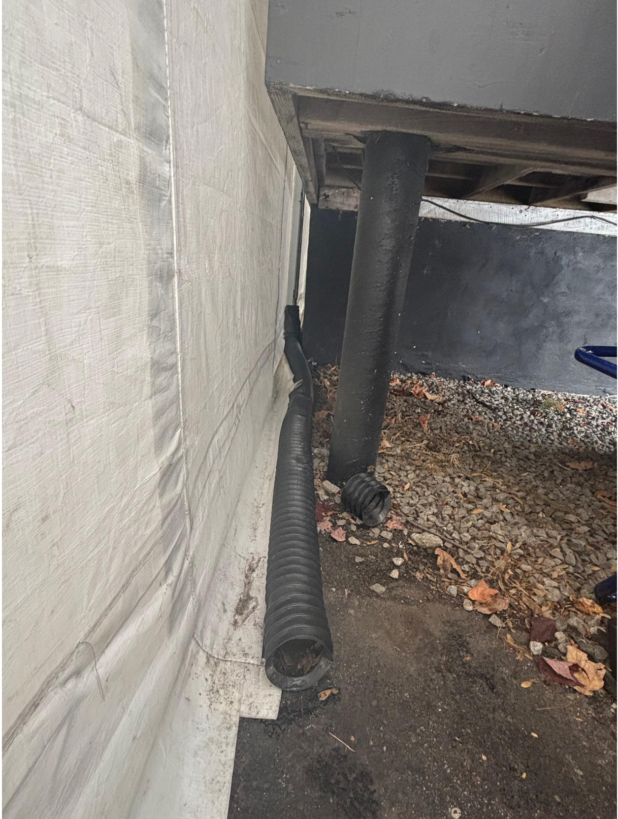
The driveway is constructed of asphalt and appears to be in fair condition. A few minor
