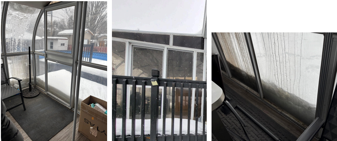
Side entrances for the solarium / sun room (1st and 2nd pictures), and joints at the bottom/flooring of the solarium / sun room (3rd picture)
