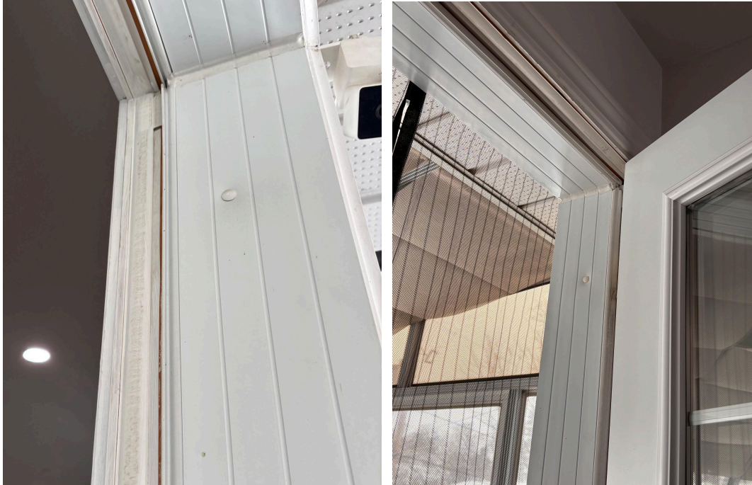
Caulking and sealant conditions at the main entrance and backdoor entrance, respectively.
